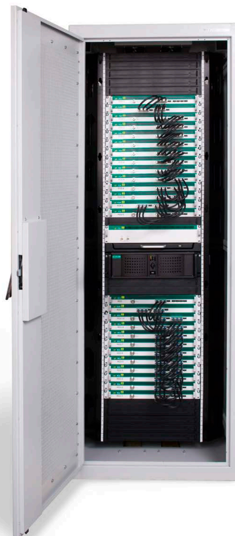
FIGURE 11: RACK INSTALLATION CONSISTING OF 11x UPLINKS, 12x DOWNLINKS AND 3x PAYLOADS
